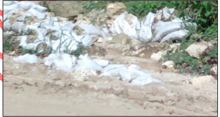
Photo 4: Sandbags poorly maintained (Photo taken by Environmental Officer, NEPA on 28 October 2014)
