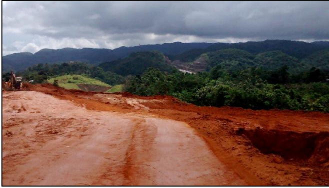
Photo 1: The start of the alignment. (K46) (Photo taken by Environmental Officer, NEPA on 28 October 2014)
