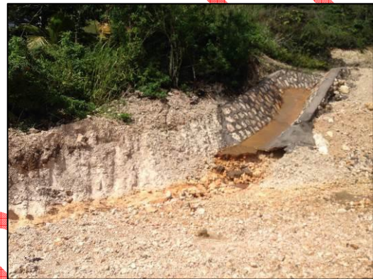
Photo 2: Drains not constructed to NWA approved designs (Photo taken by Environmental Officer, NEPA on 27 November, 2015)
