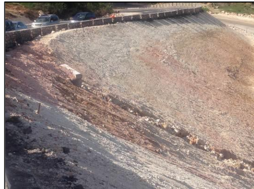
Photo 4: Cut faces with no slope stabilization (Photo taken by Environmental Officer, NEPA on 27 November, 2015)
