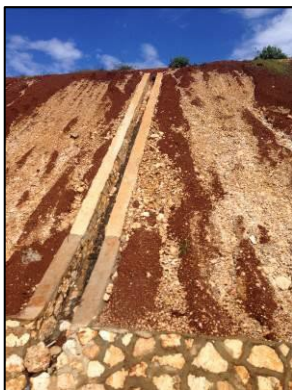
Photo 3: Cut faces with no slope stabilization (Photo taken by Environmental Officer, NEPA on 27 November, 2015)
